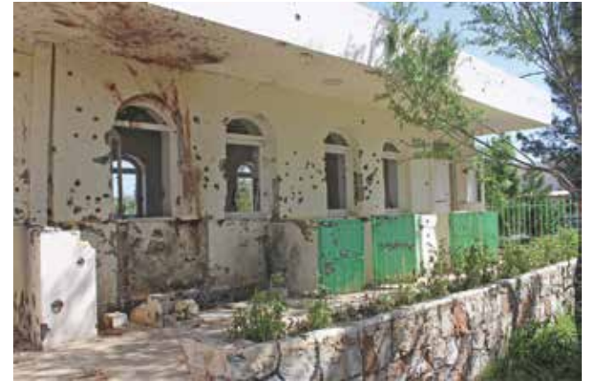
A damaged mosque near the army compound outside Mazar-i-Sharif in Balkh province after Taliban attack
